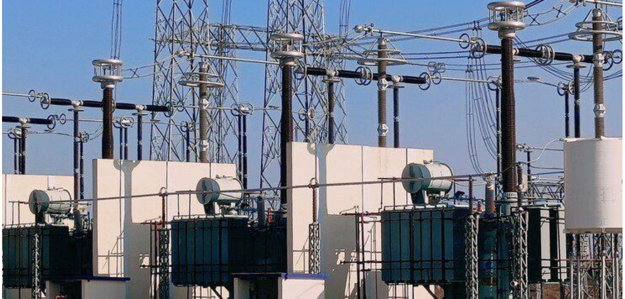
3. 765-kV shunt reactors. Courtesy: GE Vernova
