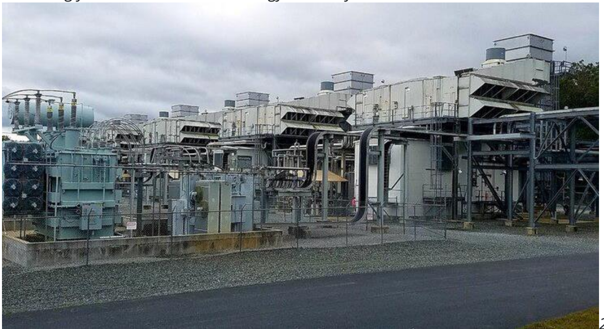
2. The Commonwealth Chesapeake Power Plant near the Virginia-Maryland border provides standby power to the local grid as well as providing synchronous condensing services and offering spinning reserve availability to the region. This was done by adding SSS Clutches to several of its GE LM6000 aeroderivative gas turbines. Courtesy: SSS Clutch
