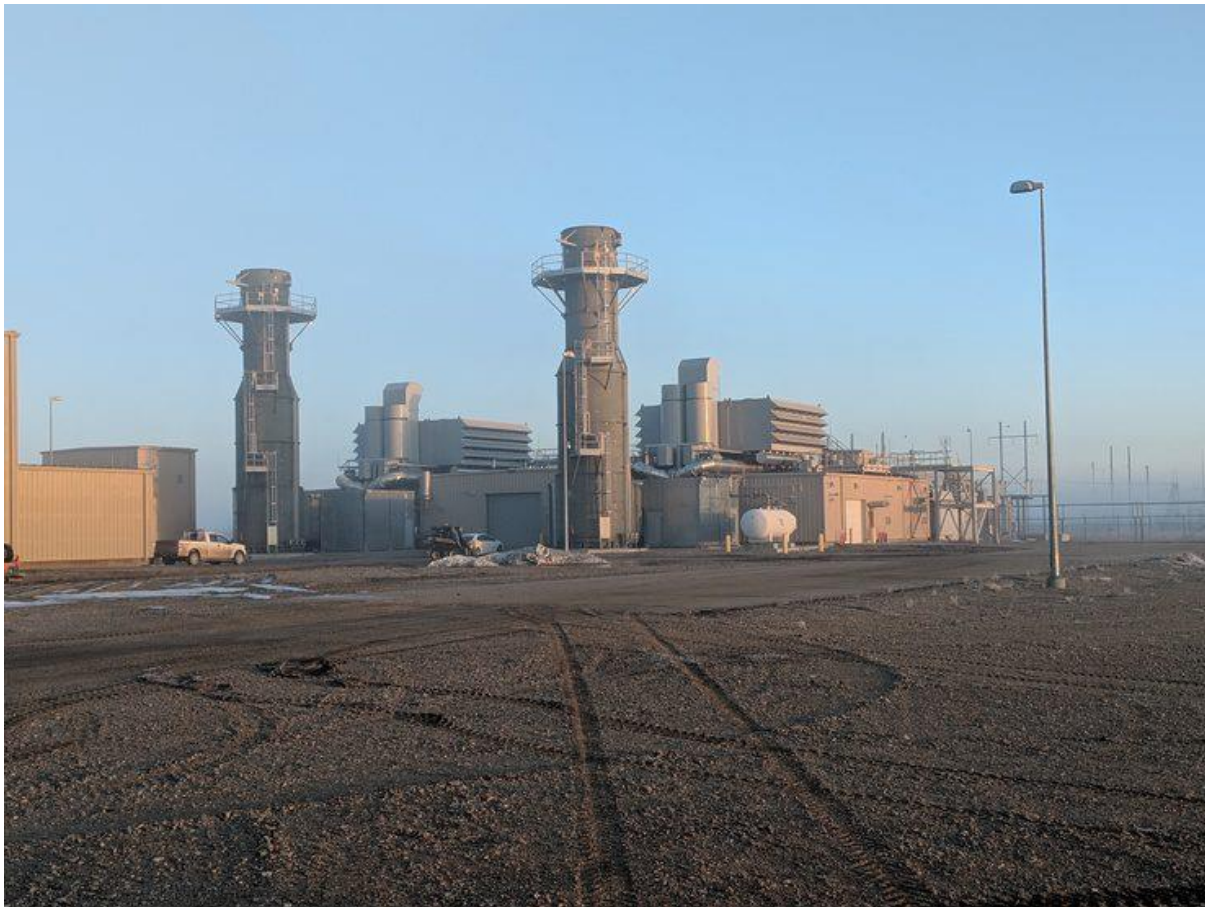
The Sask Power Ermine plant in Canada is one of many adding SSS Clutches to GE LM6000 PF+ turbines to enable them to operate as synchronous condensers. Courtesy: SSS Clutch
