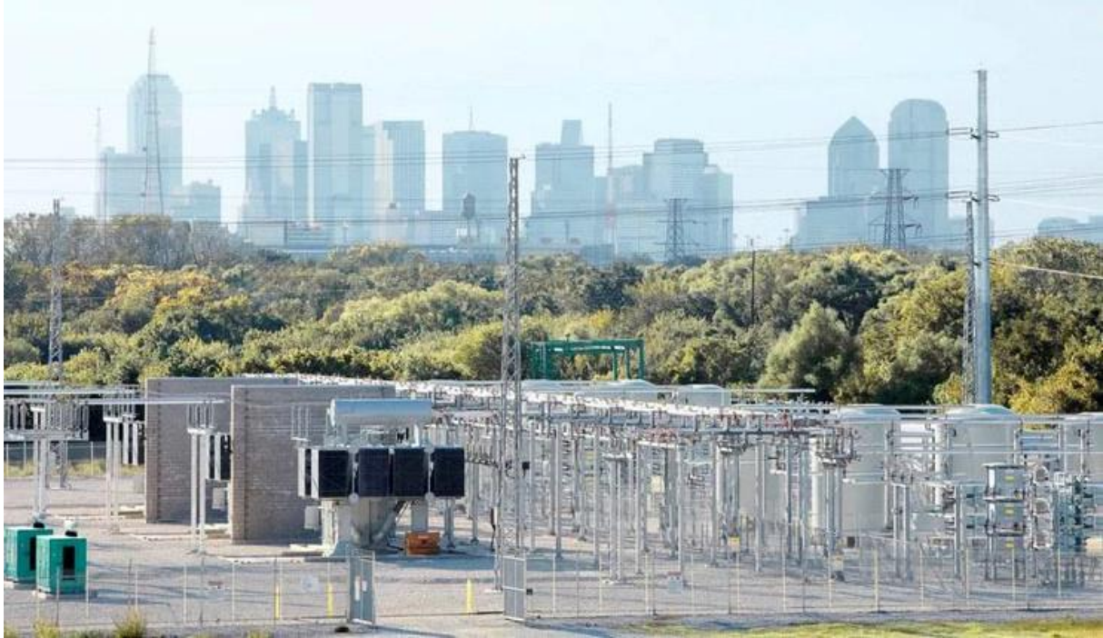
1. Static volt-ampere reactive (VAR) compensators, or SVCs, are one of many solutions used to prevent outages during times of high demand and stabilize grids that are increasingly reliant on renewable energy. Courtesy: Oncor
